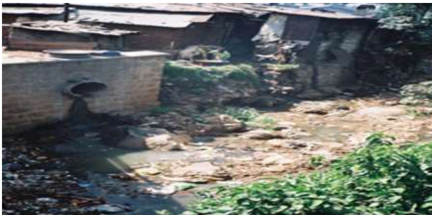
Figure 2: Discharge of liquid waste into street (Source: https://www.open.edu/openlearncreate/mod/oucontent/view.php?id=79946&printable=1 )
